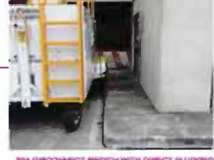
25A DISCONNECT SWITCH WITH DIRECT FLUORESCENT IN FROM (E) DIST. BD. NHF, CIRCUITS 14,16,18
