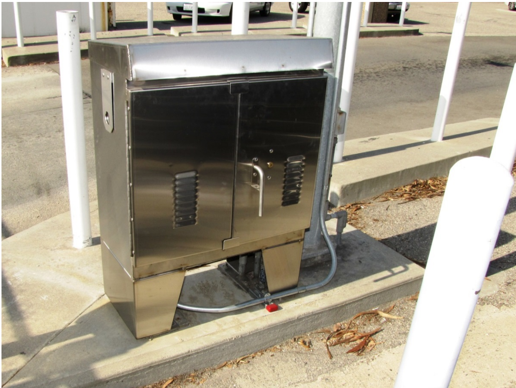
Stainless steel TE mounted on a concrete pad protected by bollards.
