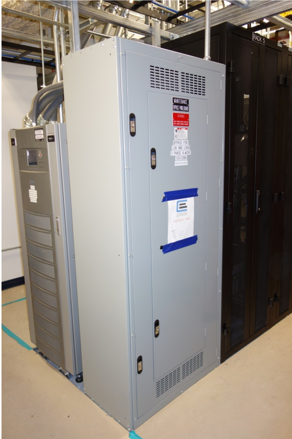
Maintenance Bypass for UPS shown.
