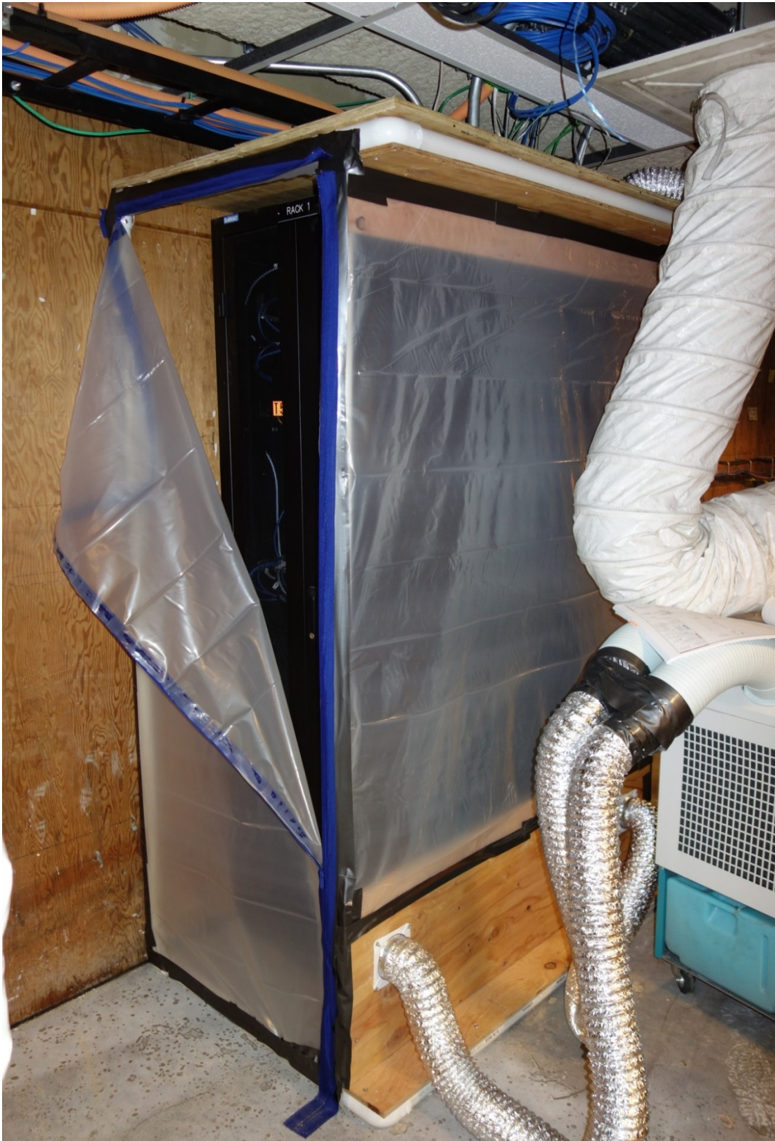
Enlargement of a cabinet protected and cooled within a fabricated PVC and plastic frame.
