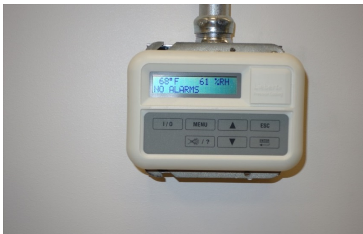
Remote monitor readout for the Liebert Site Scan unit.
