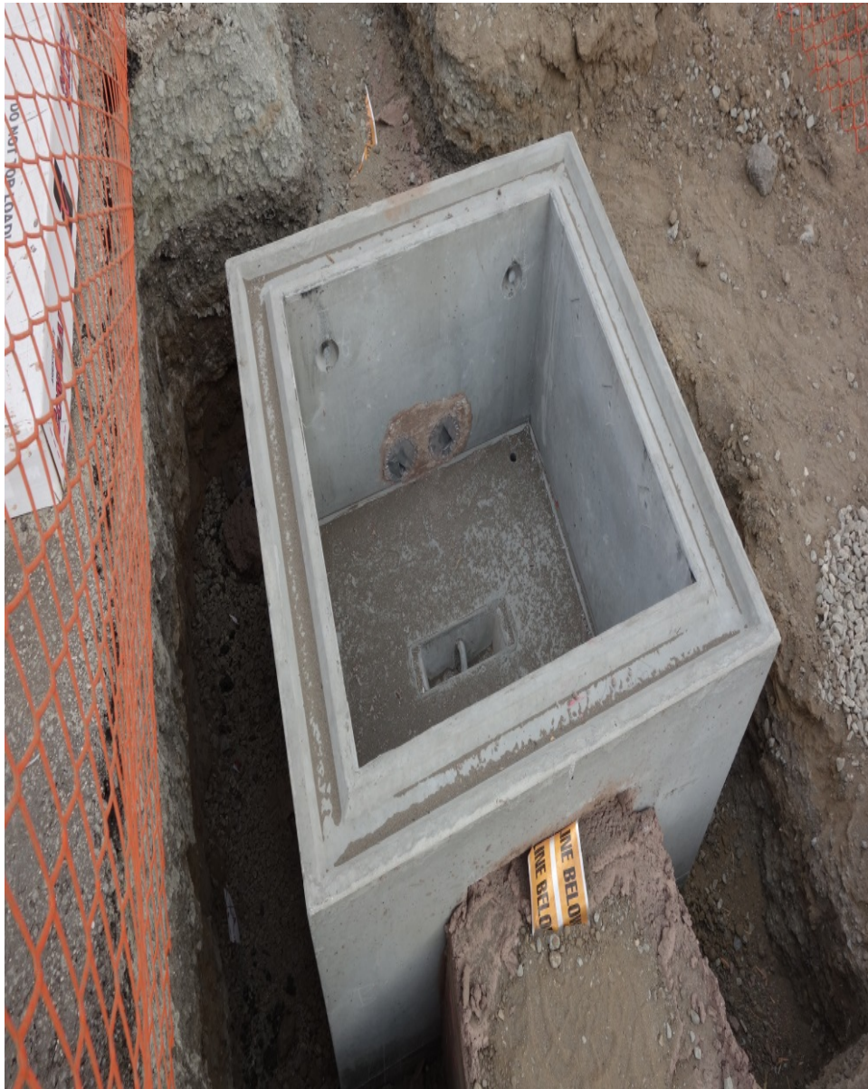
A newly installed Hand Hole for 2 entry and 2 exit conduits and awaiting cable racks.
