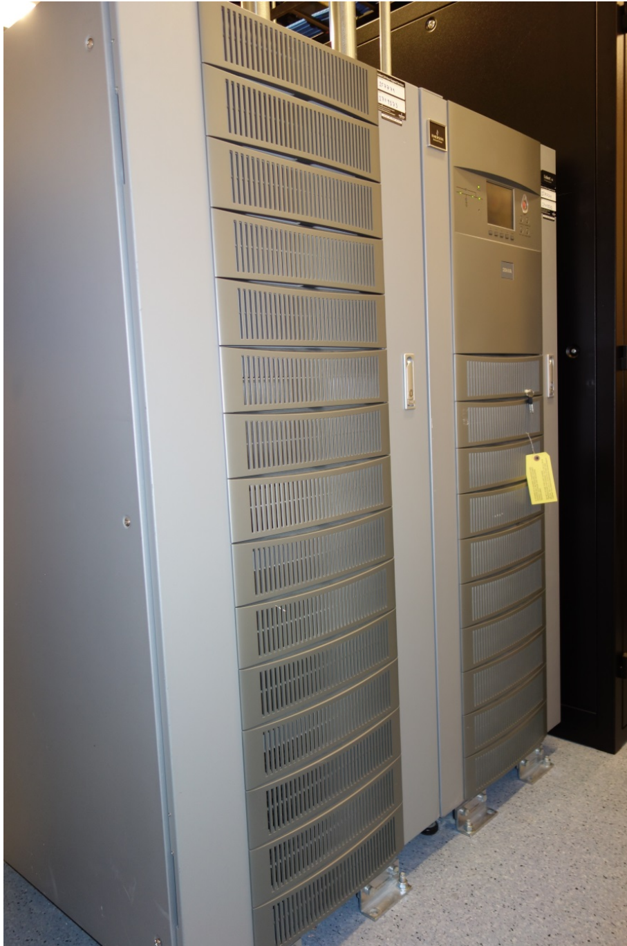
A 20kVA Liebert UPS shown with battery bank cabinet.
