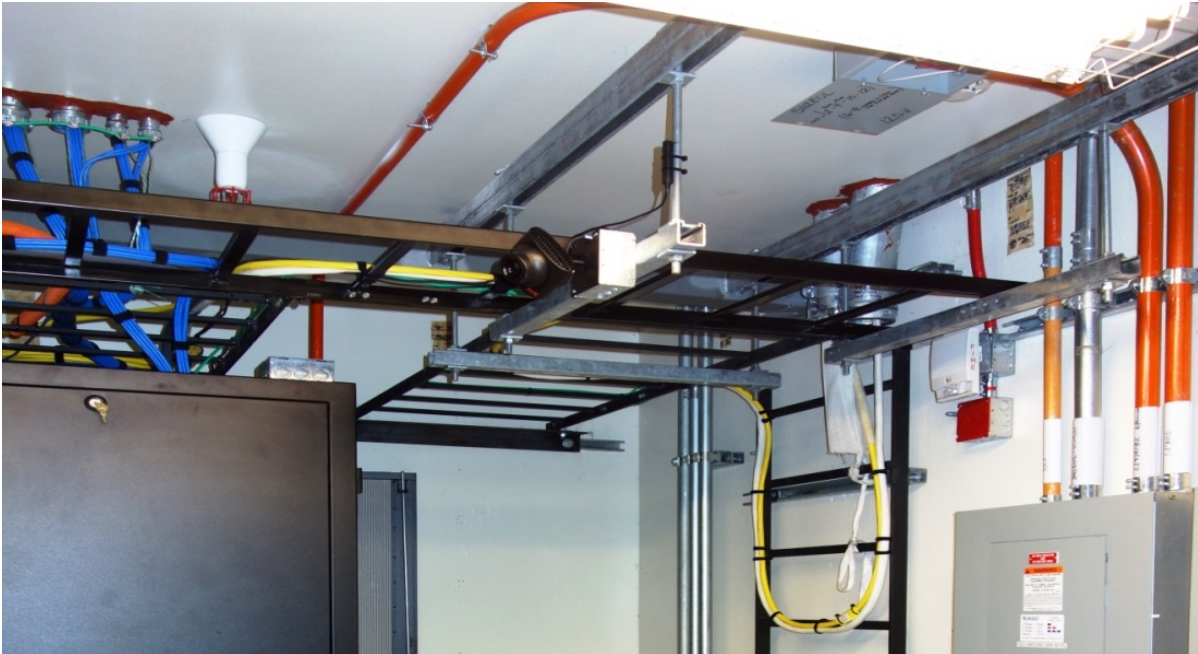
Legacy IT Room showing 8' 6" hard lid ceiling and cramped space.
