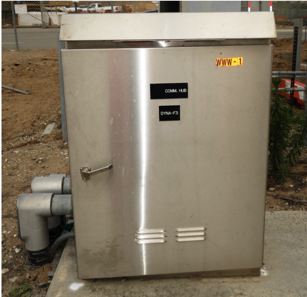
TE showing entrance and exit conduits.
