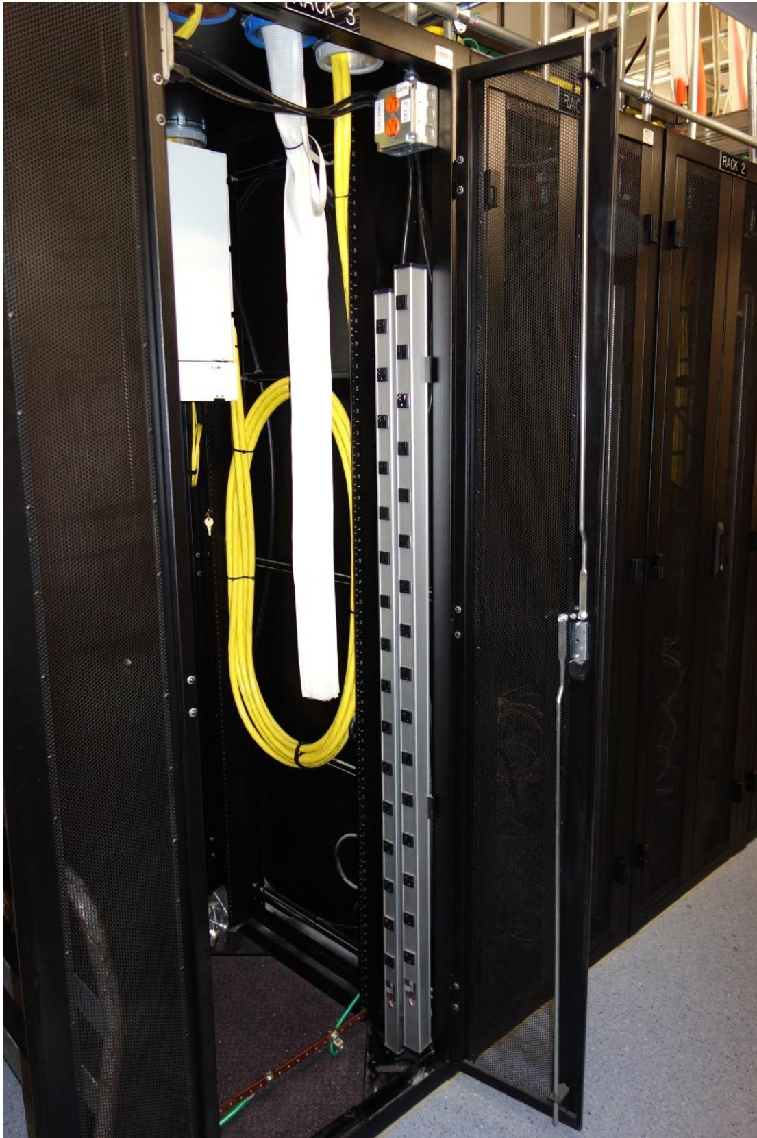
Cabinet electrical should be on only one side of cabinet rear with only one power strip.
