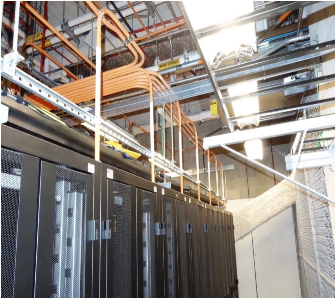
Orange electrical conduits are shown feeding individual cabinets at cabinet rear.
