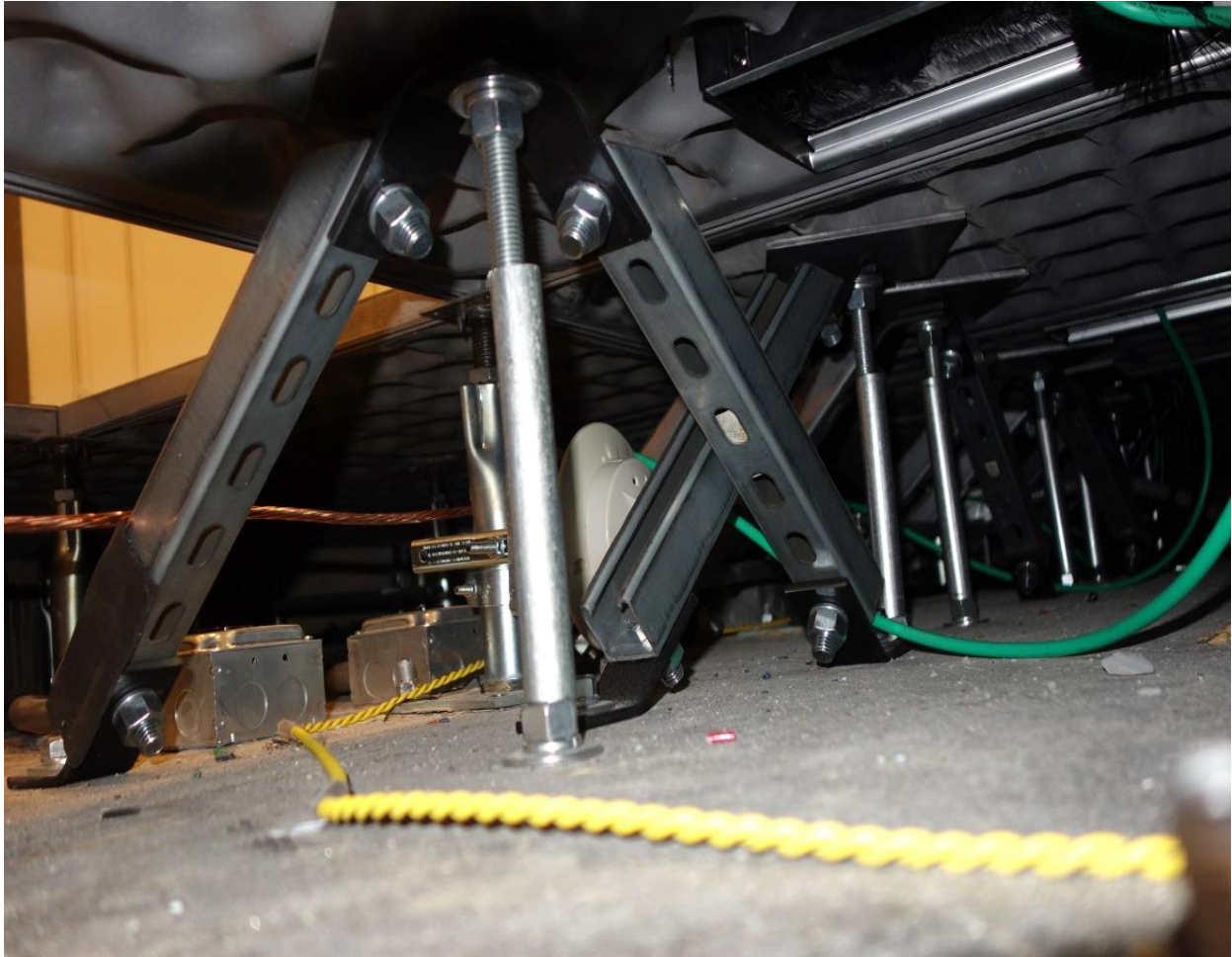
Diagonal seismic supports for equipment cabinets above a raised access floor.
