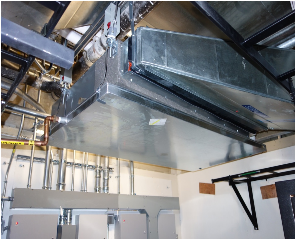
Ceiling-mount air conditioner with a fabricated drip pan and copper drain pipe.
