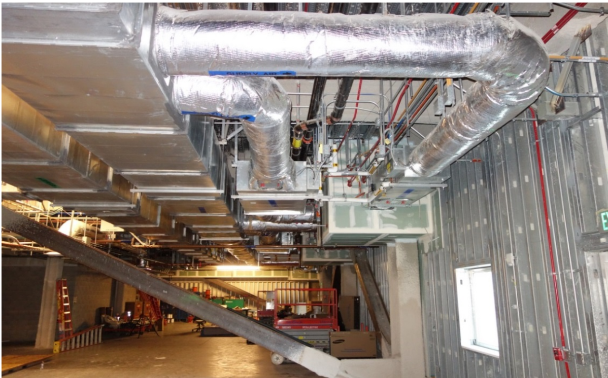
Ceiling obstructions can interfere with the pathways from IT Rooms.
