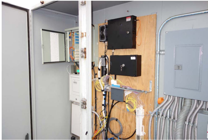
A legacy outdoor TE with plywood backboard - prior to the stainless steel requirements.
