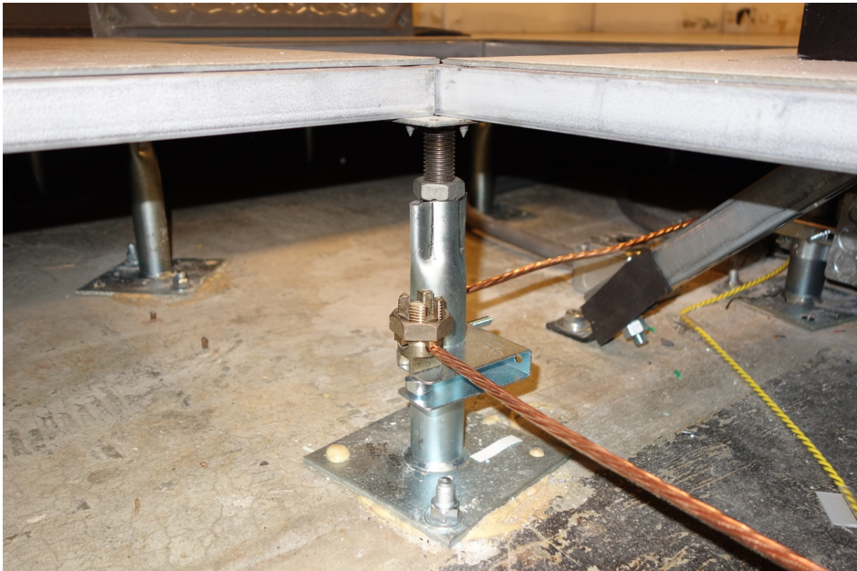
Grounding is required on raised access floors.
