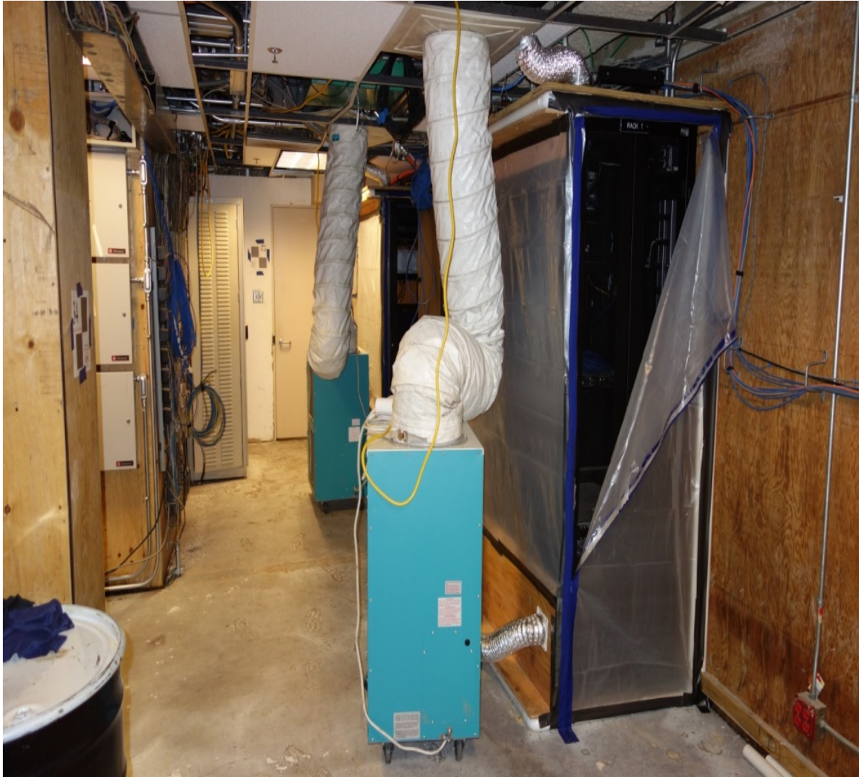
IT cabinets in construction zones shall be protected and cooled.
