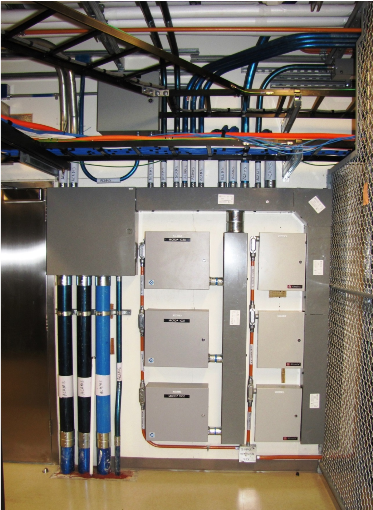
Legacy access control infrastructure installed as per previous LAWA requirements.
