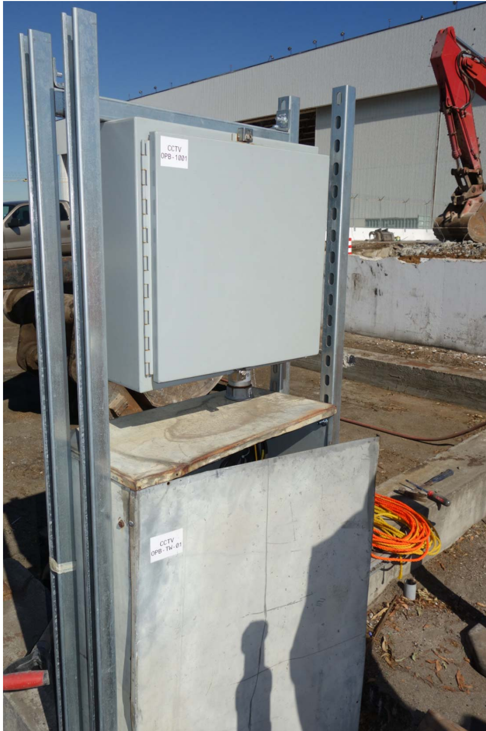
Steel NEMA 4 TE's are permitted for temporary jobs up to 12-months duration.
