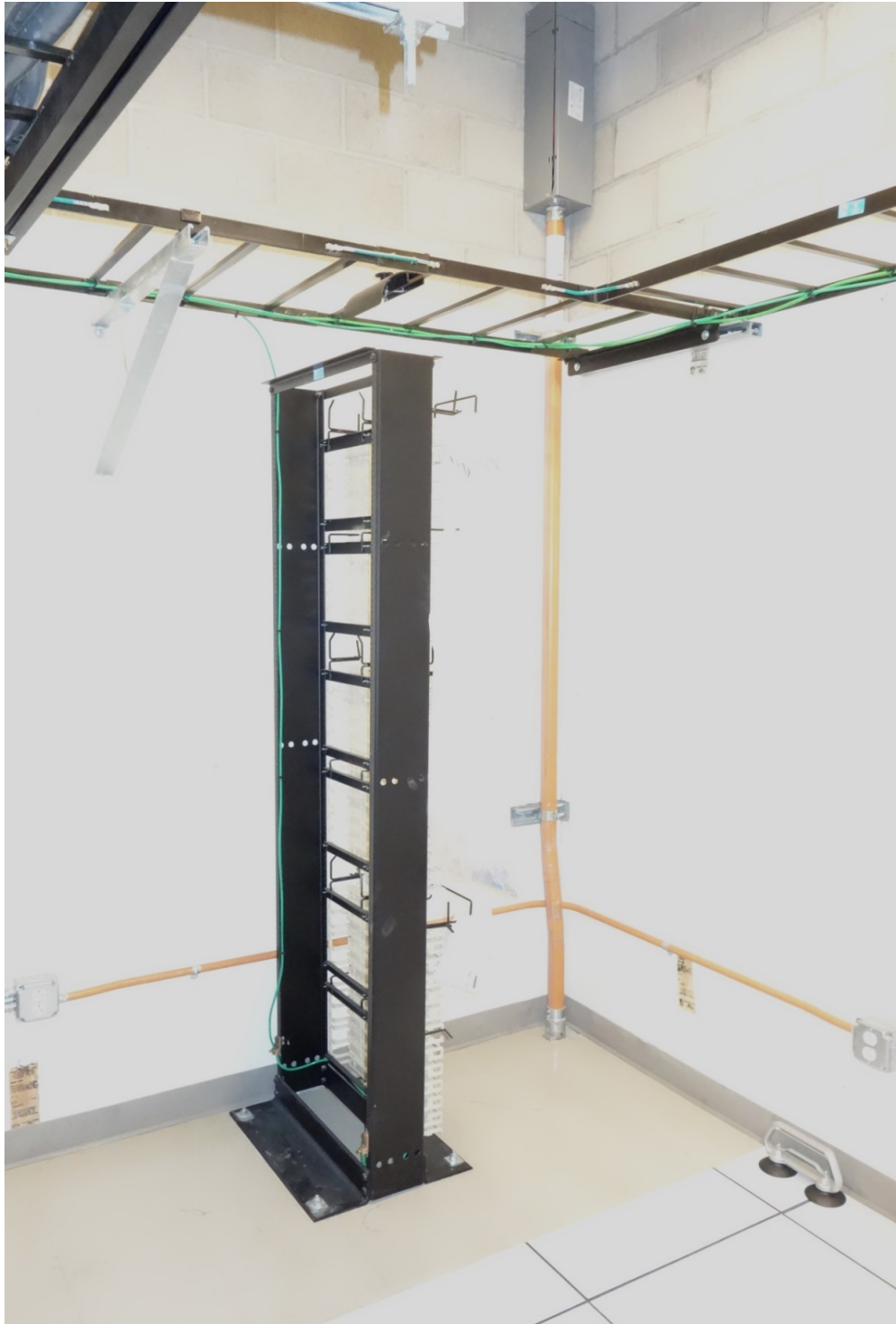
A rack for main distribution frame (MDF) expansion.
