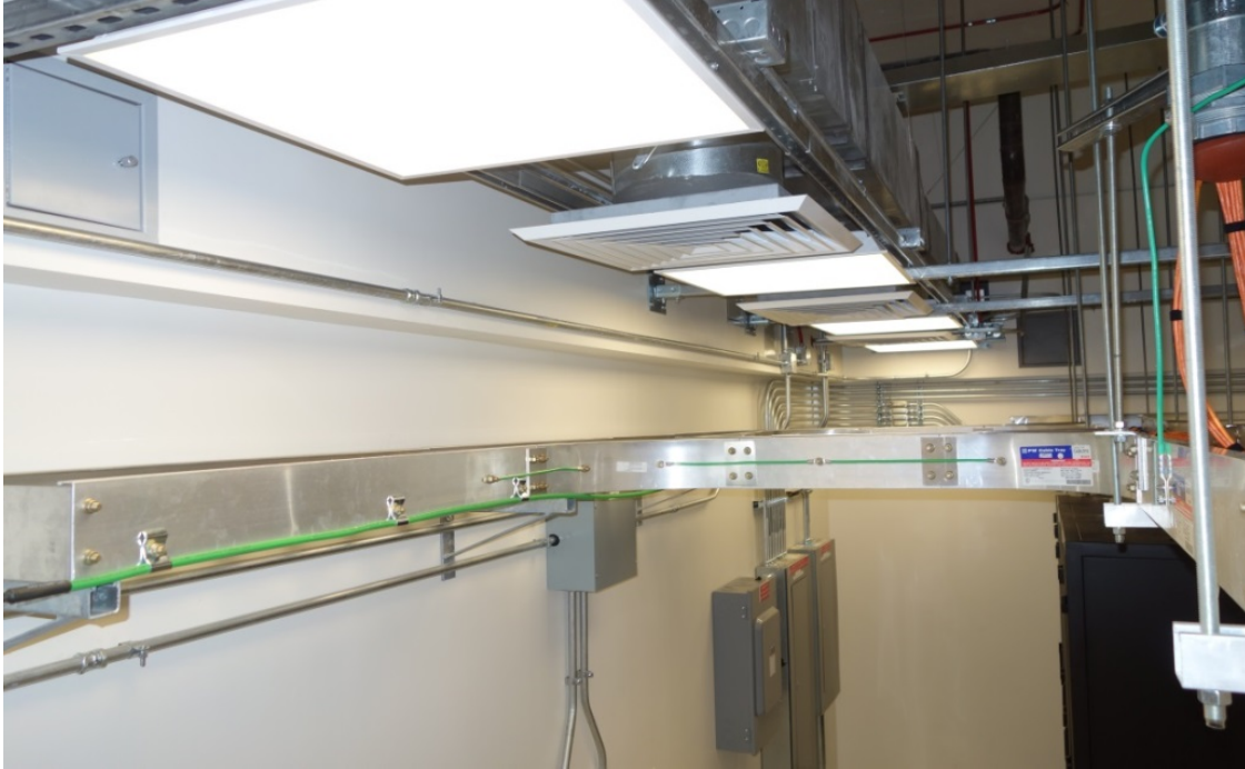
2' x 2' LED light fixtures.
