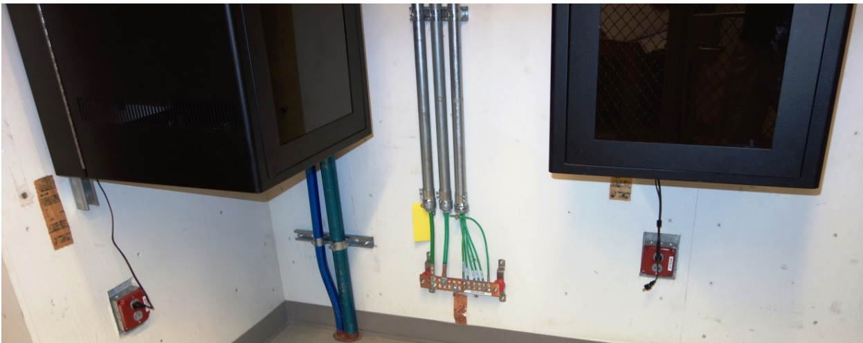
A Telecommunications Grounding busbar is required for TCWC's.
