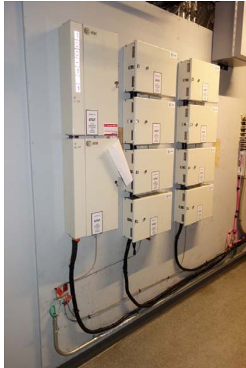
Mid-sized Copper Entrance Facility.
