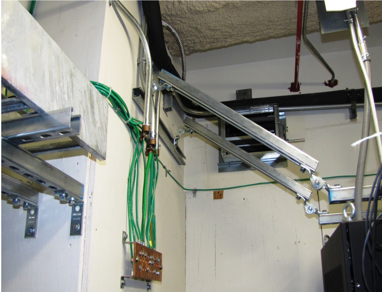
Seismic supports shown connecting to strut that supports a cable tray.
