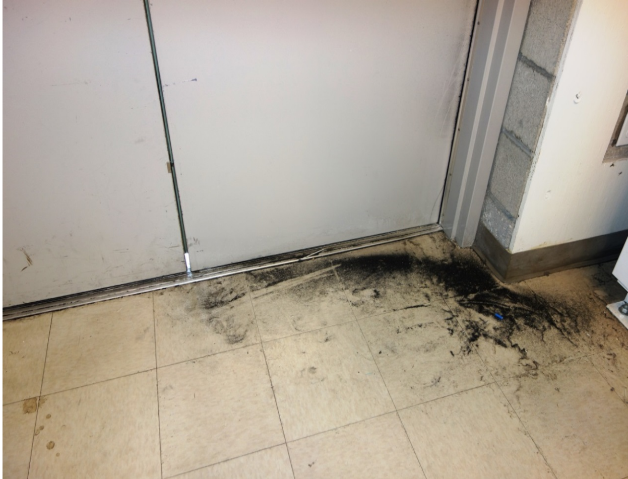
Legacy installation showing gap between doors allowing dirt inside.
