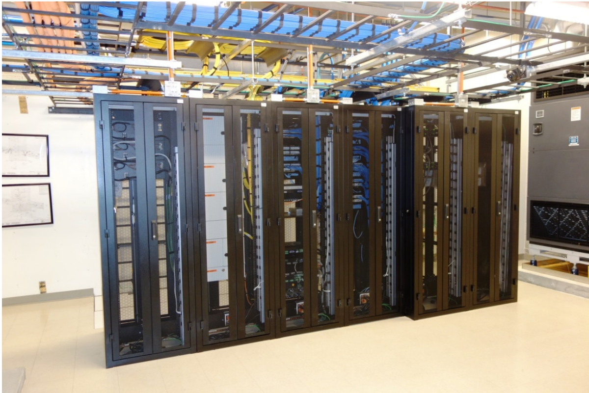
Existing IT Room shown with 1 row of Damac cabinets.
