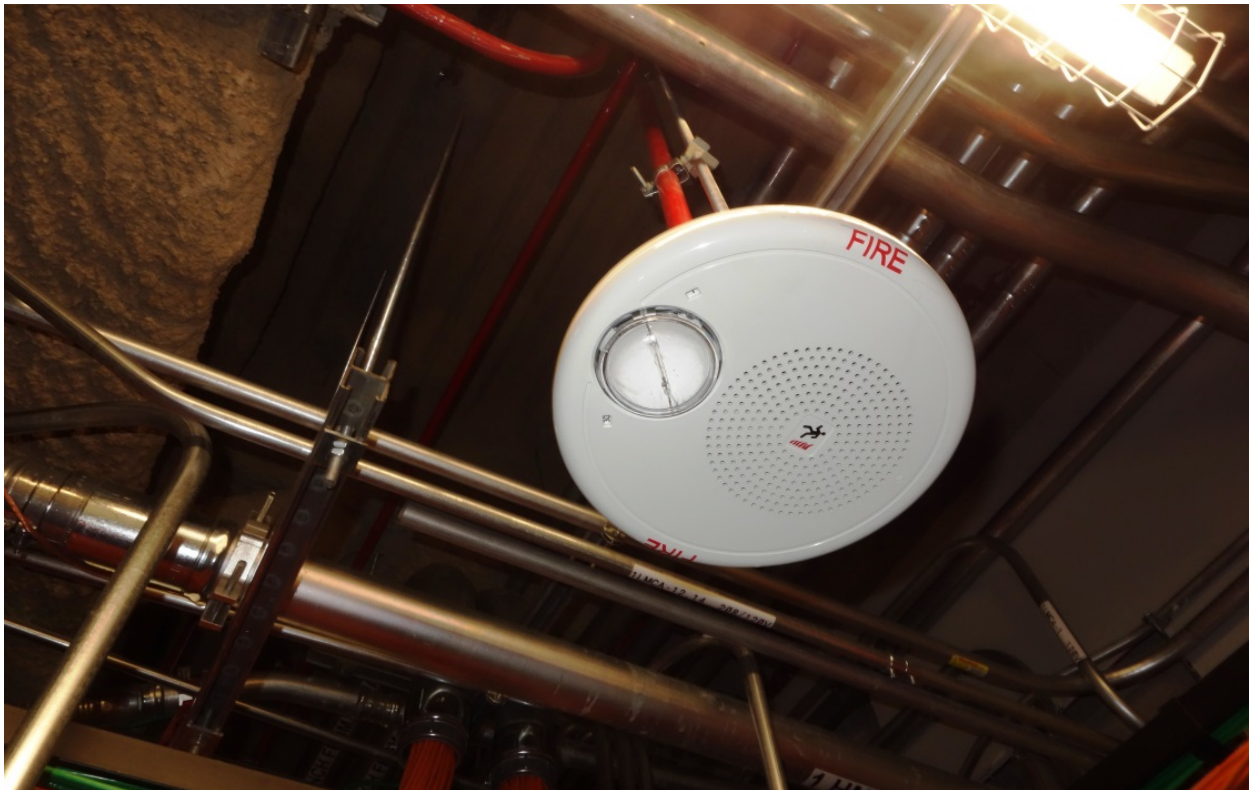
Sample IT Room smoke detector.
