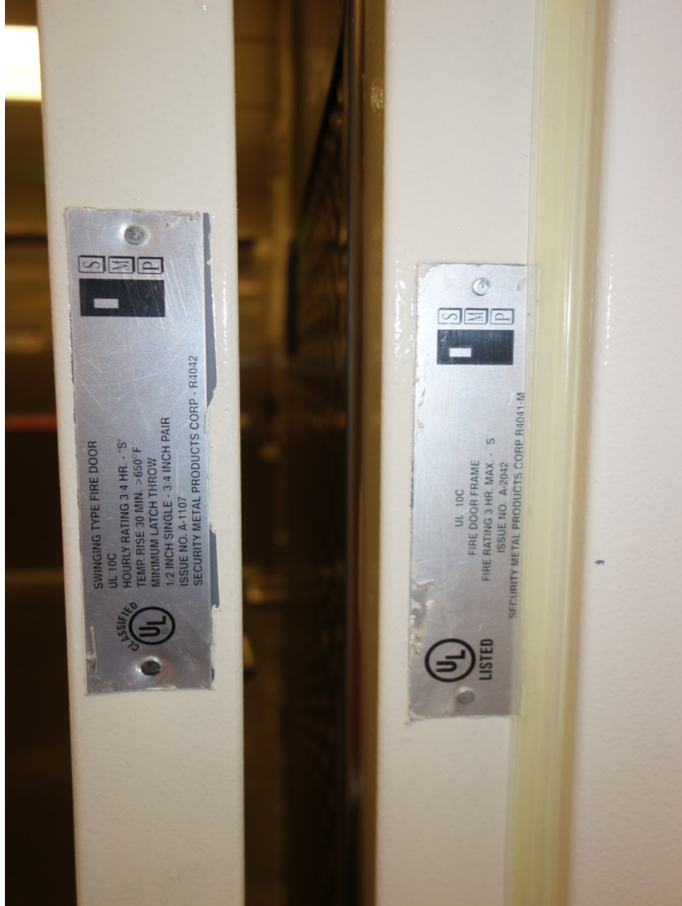
Fire protection stamp located in the inside frame of the door.
