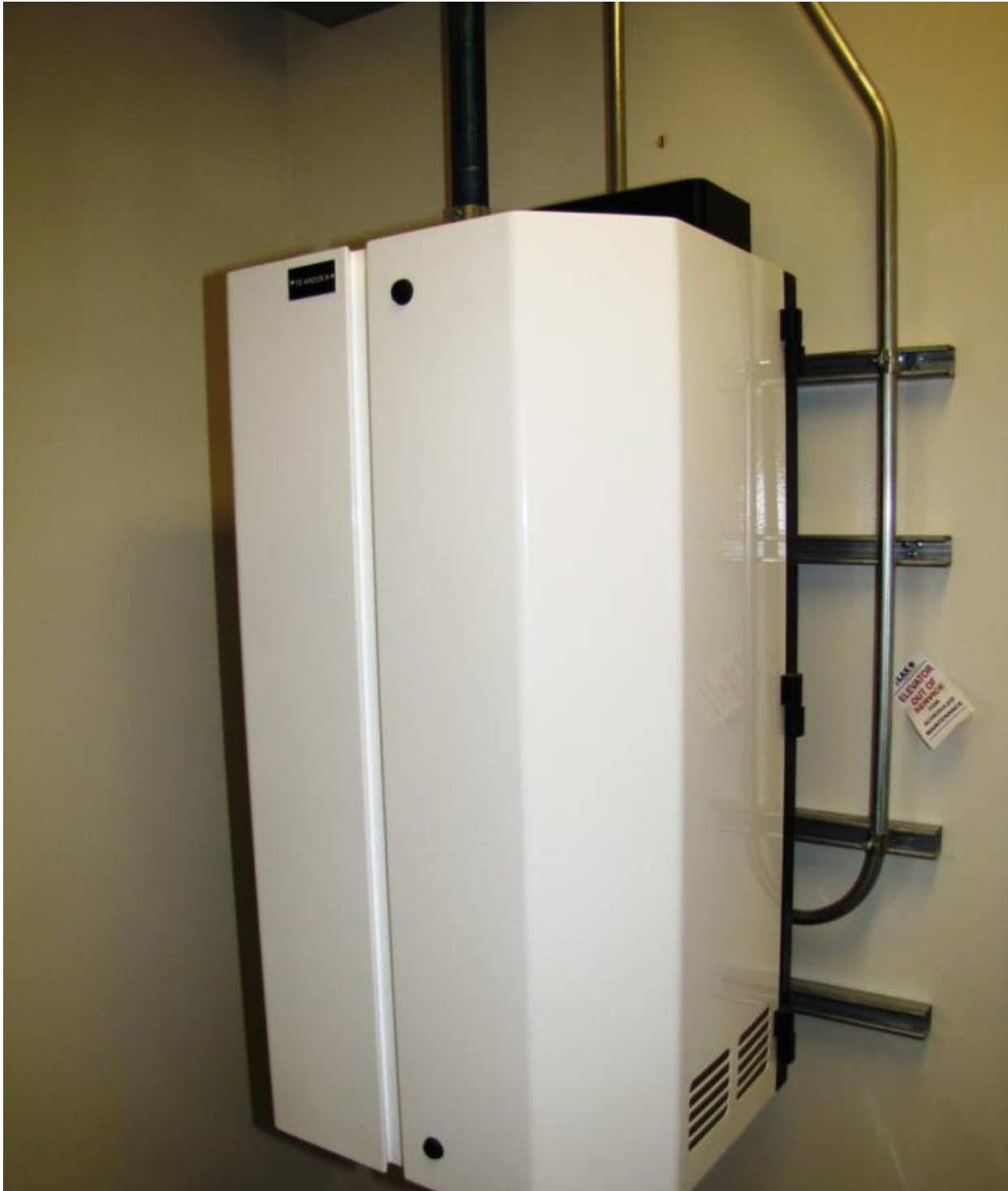
A white-colored UL-Listed Armarac TE wall-mount enclosure outside view shown.
