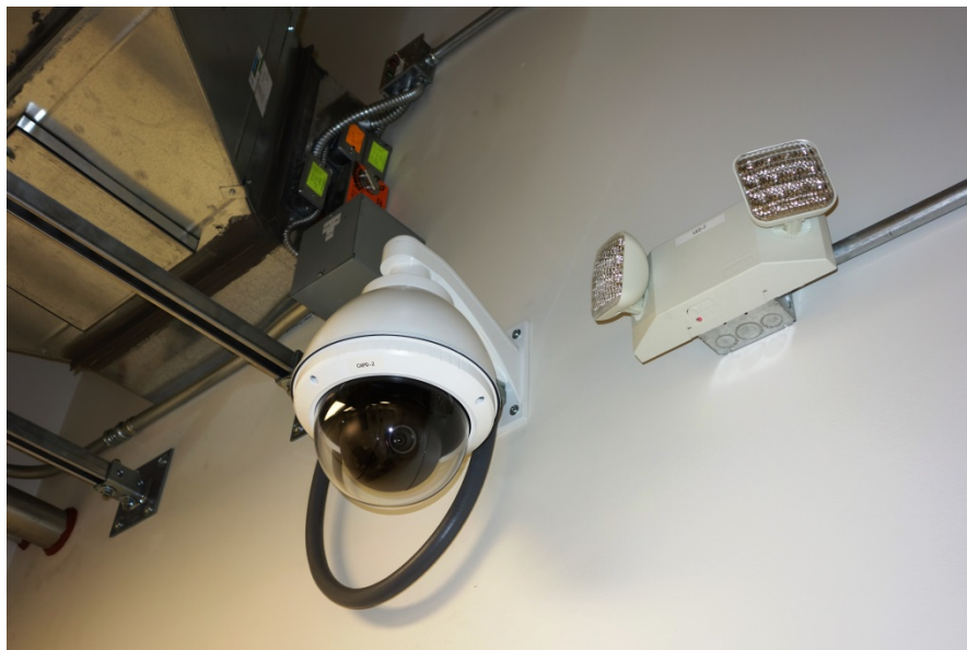
Sample Pan/Tilt/Zoom camera now used in IT rooms to replace Netbotz cameras.
