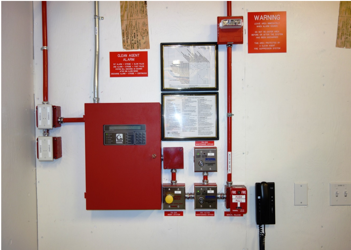
Sample fire alarm annunciator panel.
