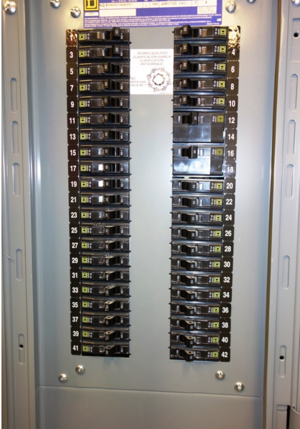
Fully populated breaker panels are required.
