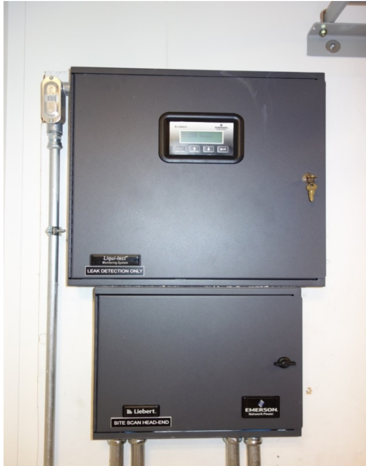
Liebert Site Scan electrical/mechanical monitoring units.
