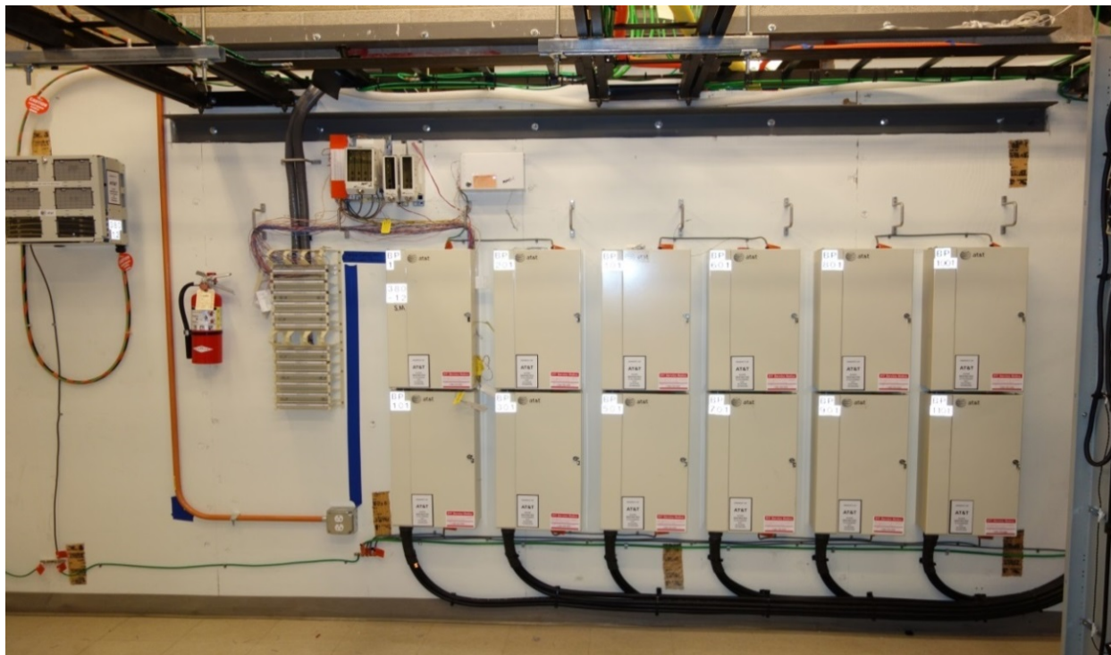
Large Entrance Facility with Service Provider-terminated cable protectors.
