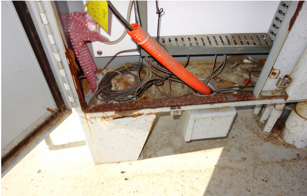
Rust is the reason for requiring outdoor TE's to be stainless steel.
