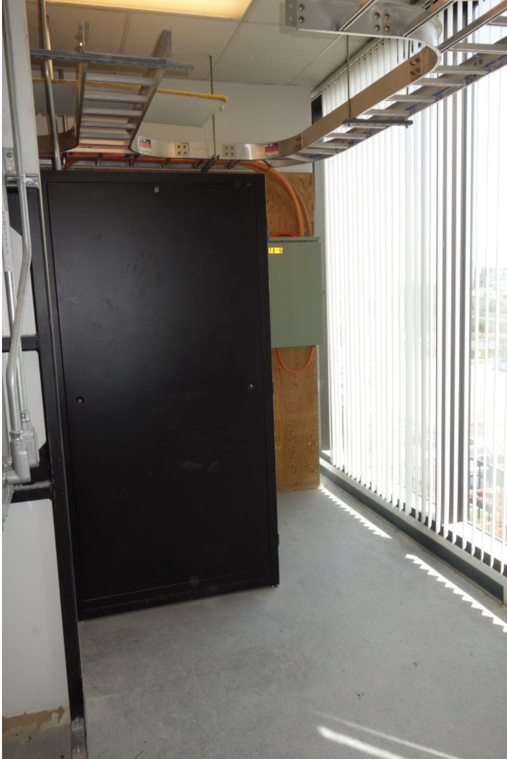
Legacy IT room showing windows.
