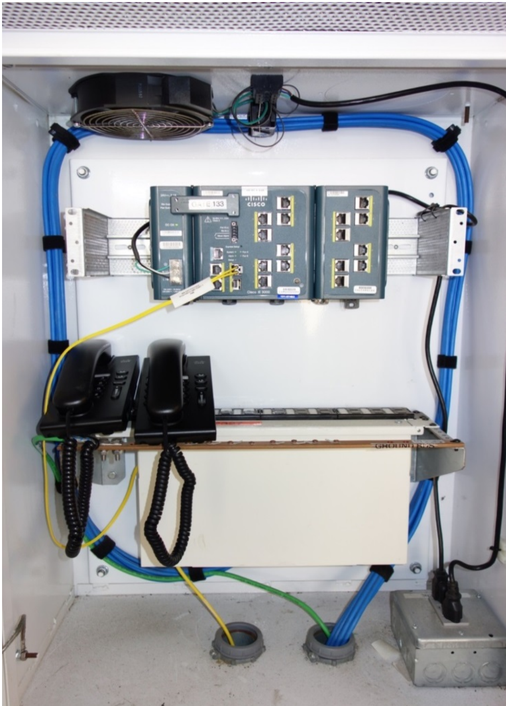
A manufacturer-provided steel backboard drilled and tapped to mount the equipment.
