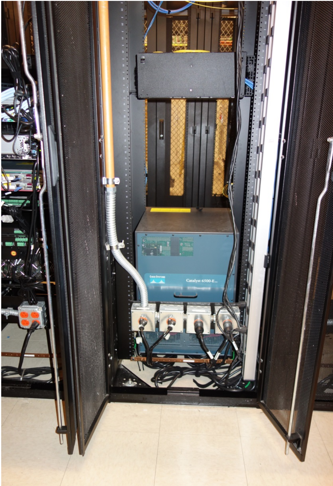
Four outlets on the bottom are ok as shown. Cabinet electrical should be on only one side of cabinet rear. One power strip should have been removed and the conduit placed on the right side.
