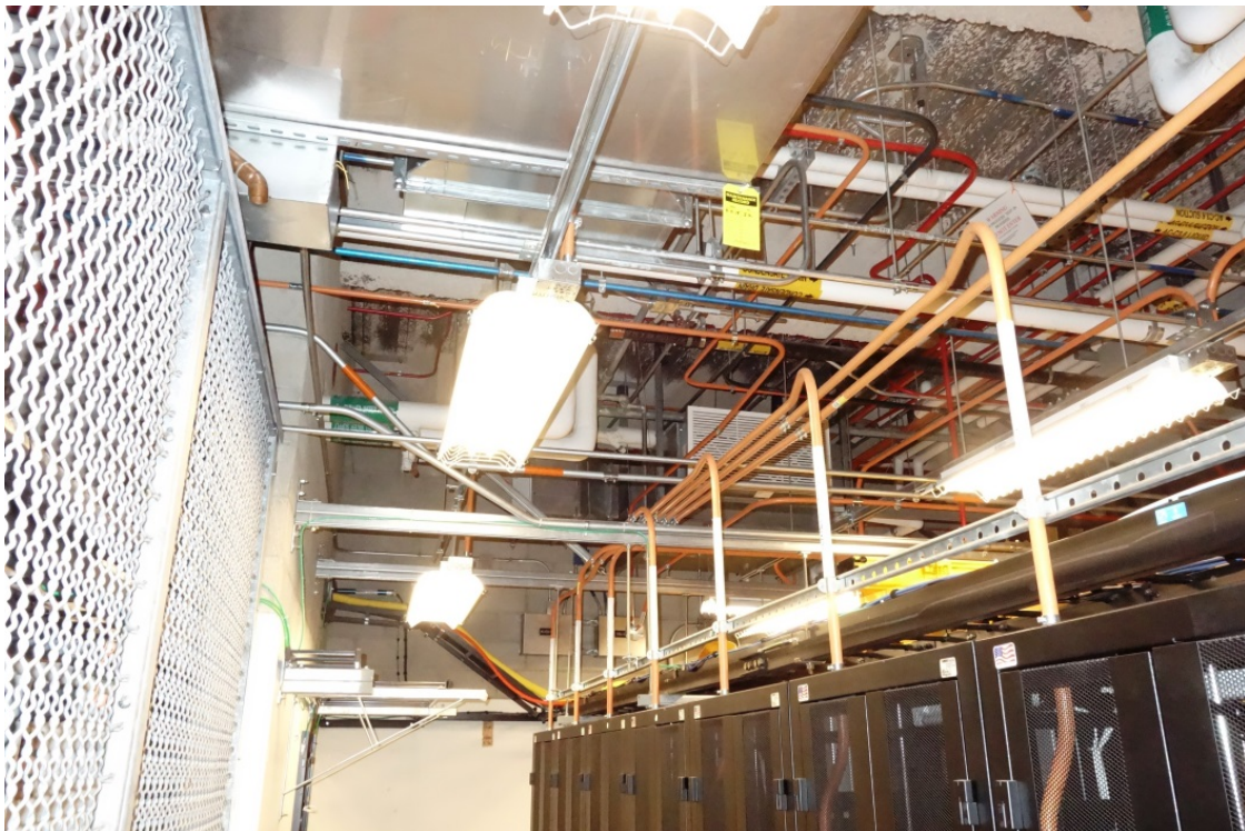
4-foot LED light fixtures.
