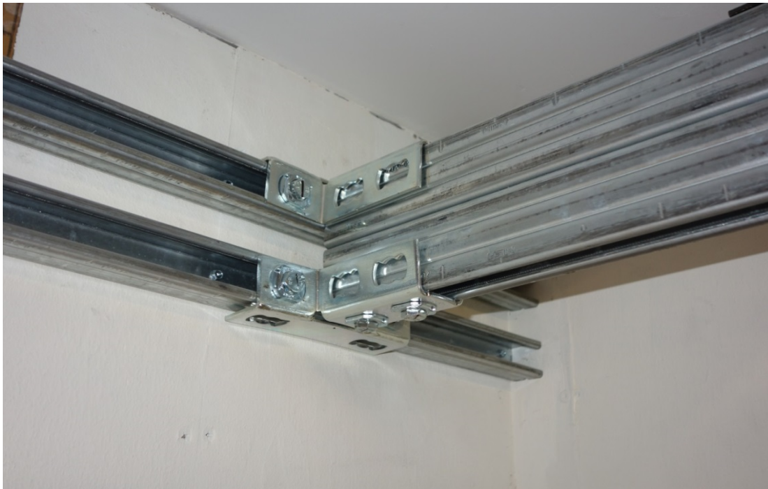
Close-up of the seismic strut framework shown anchored to wall.
