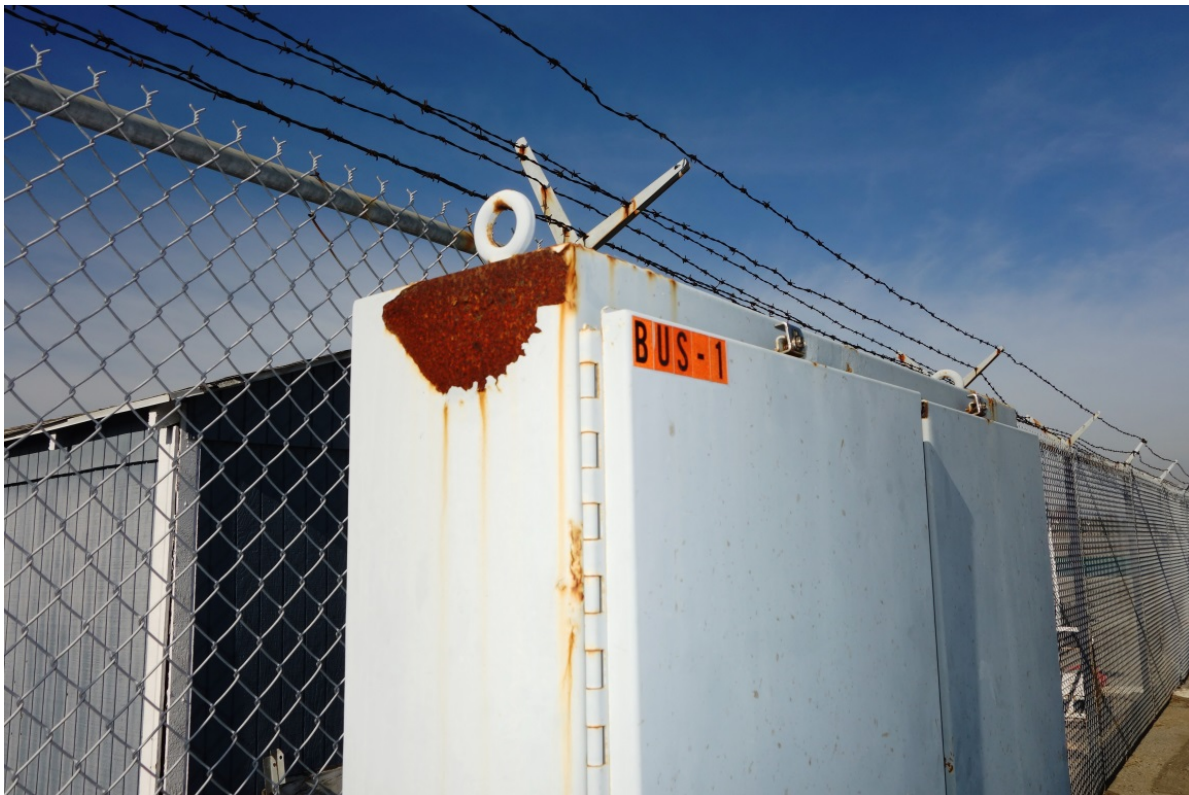
A legacy outdoor TE with appropriate labeling. Rust is the reason for switching to Stainless Steel.
