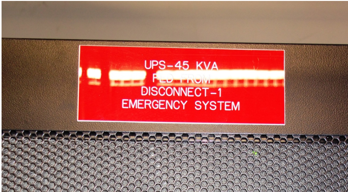
Calculated load for this MPOE required a 45kVA UPS.
