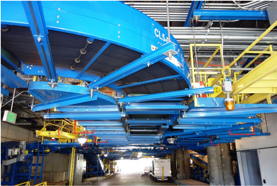
Another sample of ceiling obstructions.
