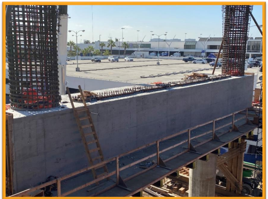
The same work area with concrete now poured as of Monday, May 4
