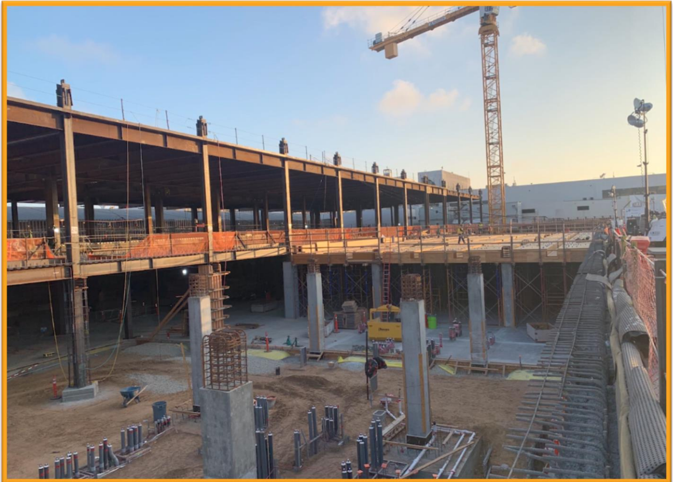
Above: Foundation work and steel erection, pictured airside, help the future Head House building take shape
