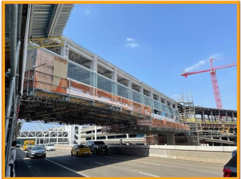
Glass panel installation is ongoing on the pedestrian bridge structure between Terminals 4 and 5
