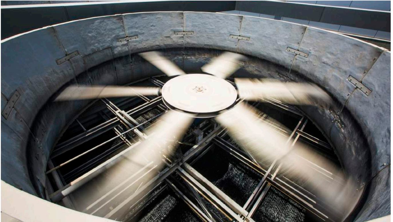
Hamad International Airport cooling plant
