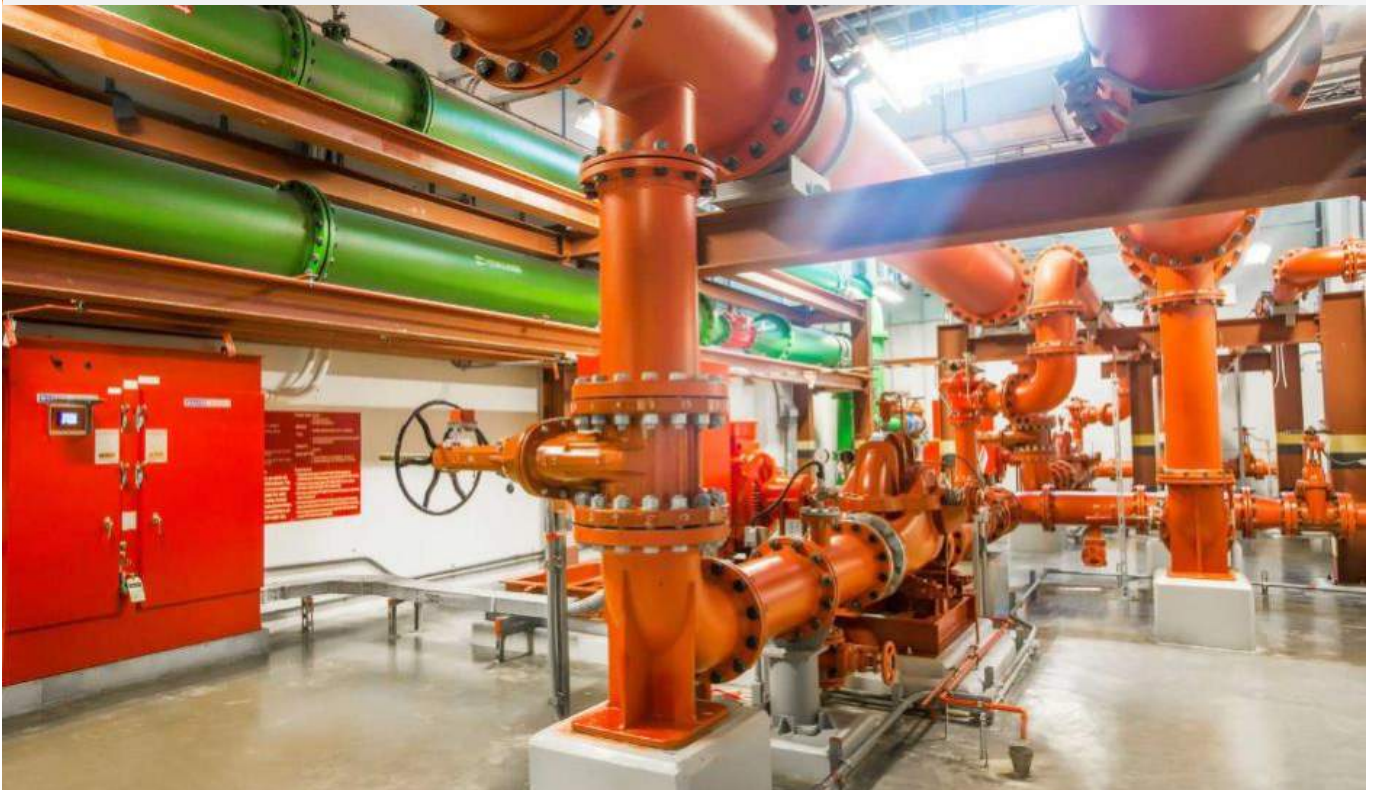
Hamad International Airport fire water system
